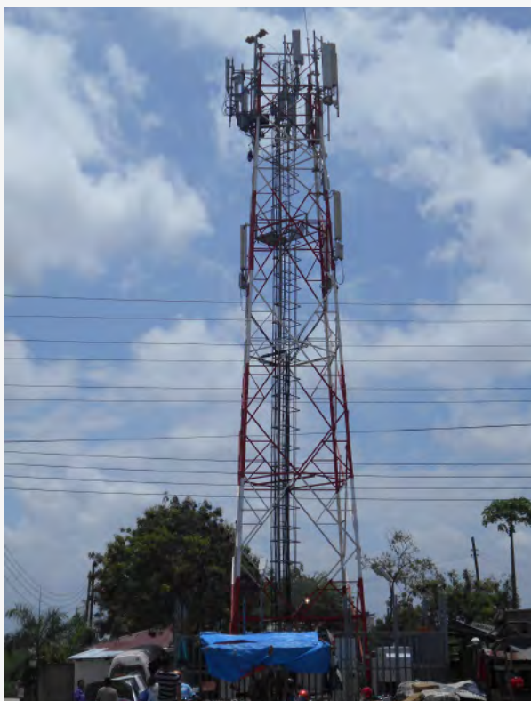
A base station at Magomeni Usalama, Dar Es Salaam.
